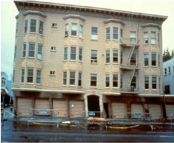
Figure 6:6 Compromised First Story
